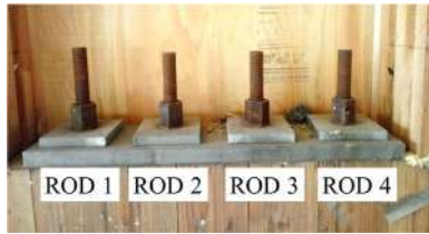
Fig. 7. Rod numbering convention for post-tensioned shear walls in a construction access window.
